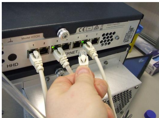
Figure 23 - Router for ACQUITY UPLC connections
