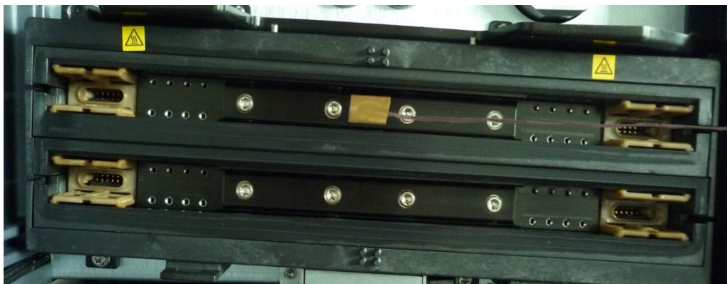
Figure 4 Installing the thermometer probe in the CM-A:
