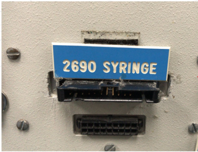
Connectors Broken & Replaced
