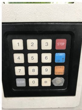
Keypad Not In Good Condition
