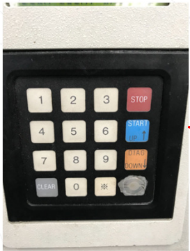
Keypad Not In Good Condition
