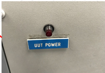
UUT Power Light Indicator Not Work
