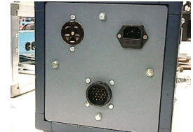
Old Power Panel
